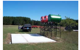
Proper fuel tank signage & loading pad
